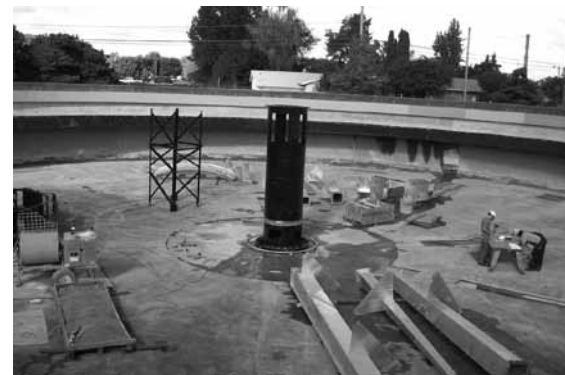
Capital improvements provide capacity for community growth
