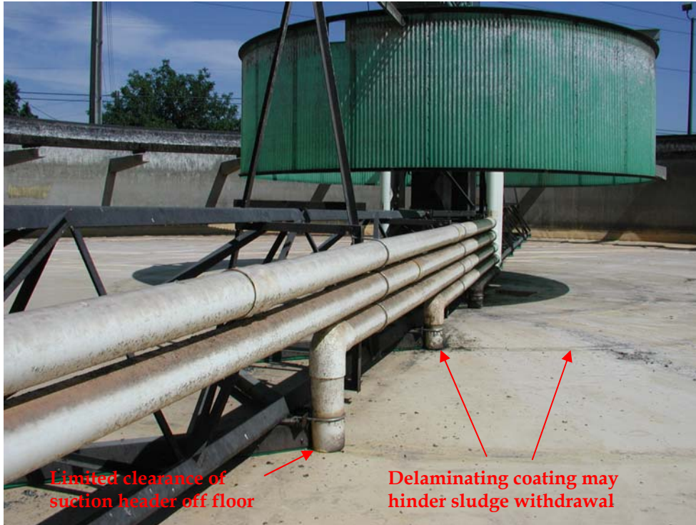
FIGURE 3 Existing Secondary Clarifier Suction Headers MMMC Facility Plan, Eugene-Springfield
